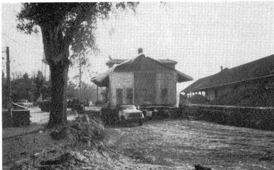
One-half of the Passenger Depot arrives at its new home next to the old freight depot which is also part of the Museum-Park Complex.
